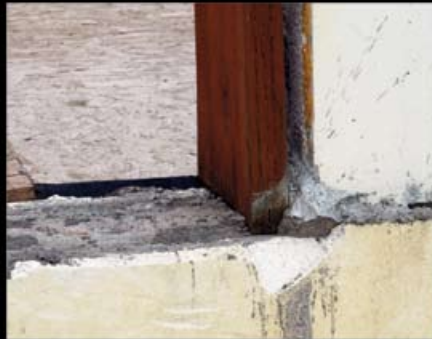
Wood Cups & Leaks In just three months the "new" treated lumber will corrode improper fasteners.
