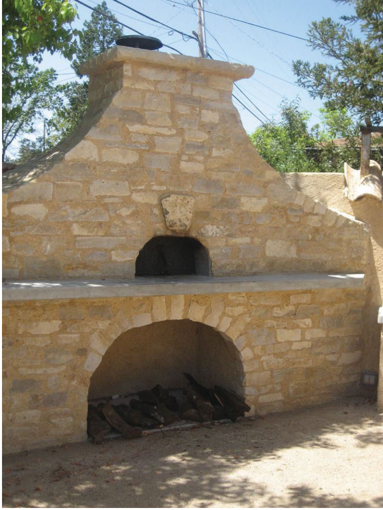
An outdoor fireplace and pizza oven — also faced in Oakfield Weather Edge Thin Veneer — were put in place so that dinners, conferences and outdoor education sessions can be held in the courtyard.
